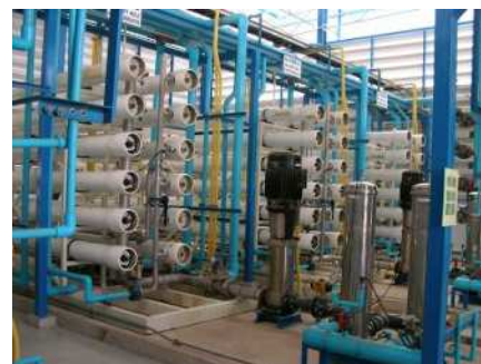
THAILAND: Amata City Industrial Estate Water Reclamation Treatment Plant 9,000t/day and 6,000t/day
