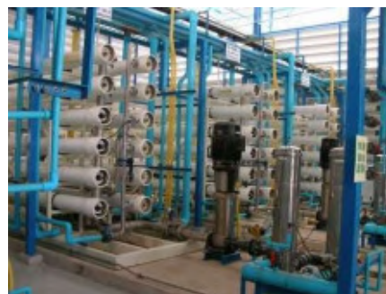
THAILAND: Amata City Industrial Estate Water Reclamation Treatment Plant 9,000t/day and 6,000t/day
