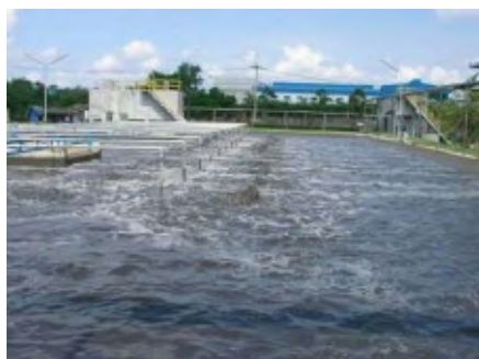
THAILAND: Amata City Industrial Estate Wastewater Treatment Plant 12,000t/day
