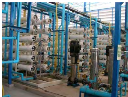
THAILAND: Amata Industrial Estate Water Reclamation Treatment Plant 6,000t/day
