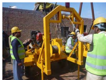
パキスタン国グジュランワラ下水・排水能力改善計画 The Project for Upgrading of Mechanical System for Sewerage and Drainage Service in Gujranwala (Pakistan)
