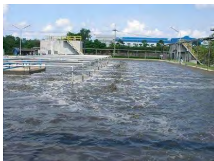
THAILAND: Amata Industrial Estate Wastewater Treatment Plant 12,000t/day
