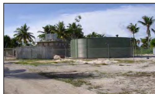
Kiribati Aeration Tank & 400 ton Reservoir
