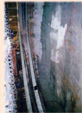
Stabilized ground by Jet Grout just before launching of tunnel boring machine
