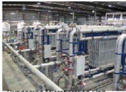
Bundamba Microfiltration Unit
